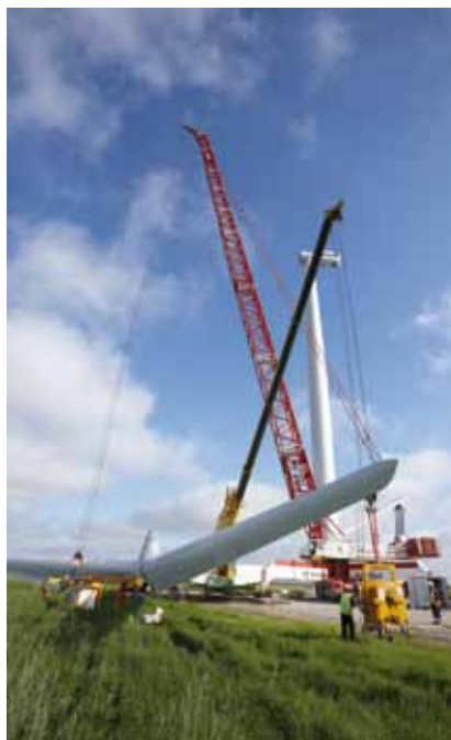
The Vattenfall electricity company, which is the largest owner of Danish onshore wind turbines, was also responsible for the largest project under the scrapping scheme at Nørrekær Enge, where 77 older wind turbines were replaced with 13 x 2.3 MW turbines. In the photo, the installers are setting up one of the new wind turbines, which were connected to the grid in 2009.
